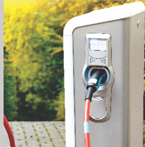
ELECTRIC CAR CHARGING STATION
